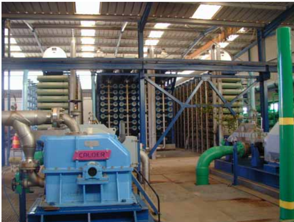
Train 2 at the Agragua, Spain, seawater reverse osmosis facility (shown as the middle train in the background of this photo) was retrofitted with FILMTEC™ spiral wound elements. The high pressure pump is shown in the foreground. (Photo courtesy of Agragua Desalination Plant)
